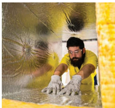
Insulation impaled through welded pins
